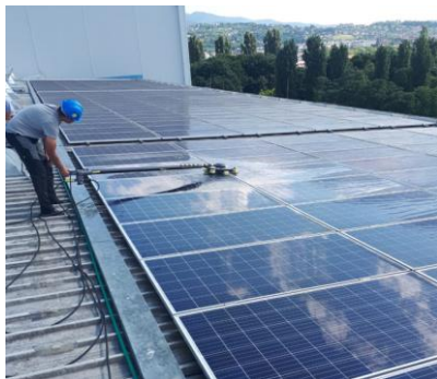
Solar power plant on the roof of the building
